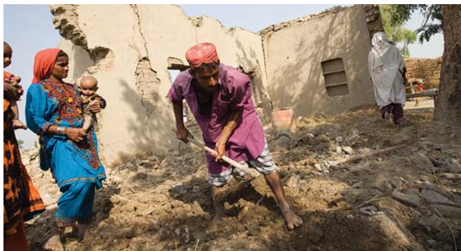
3.4 Building damage, Pakistan 📷 Marco Botelli/IOM Pakistan.
